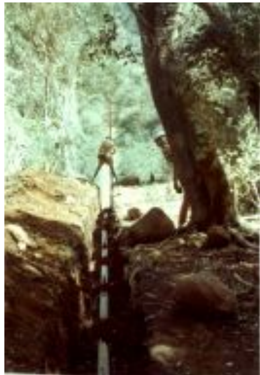
Kifufu pipeline running through the forest
